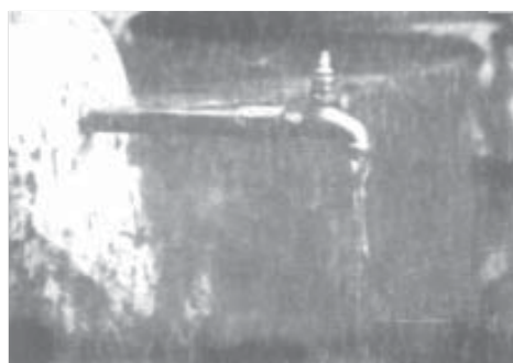
Leaking Brass Tap
